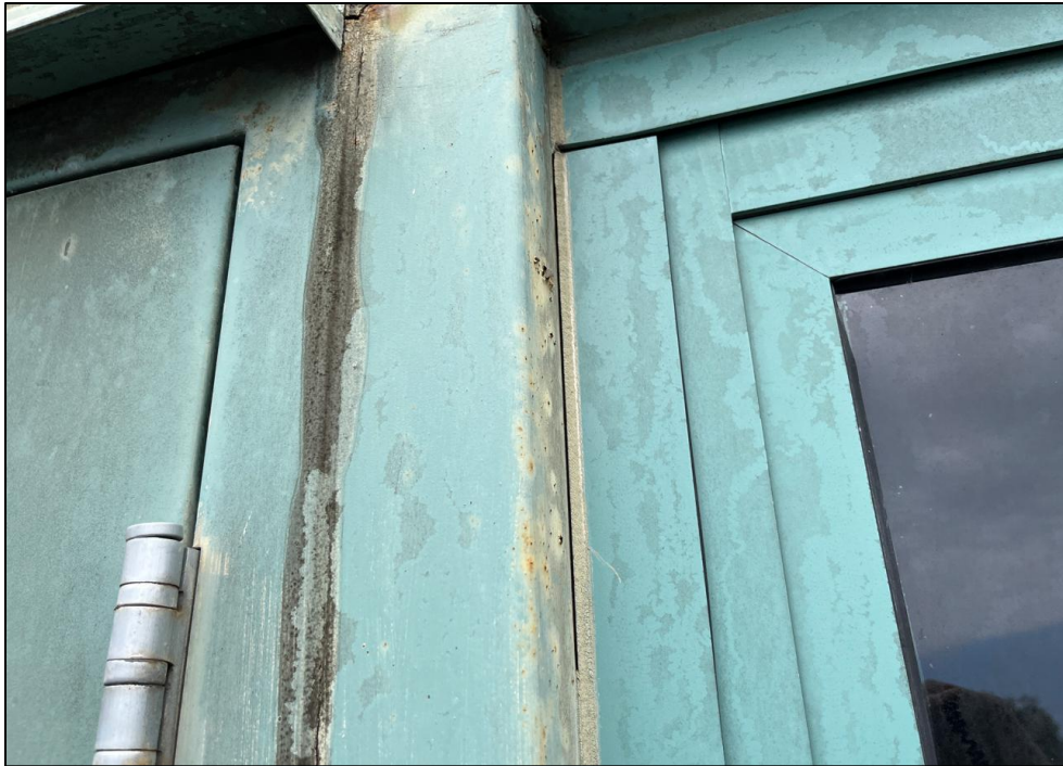
Photo 14 - Interface of aluminum windows and steel door frame at west elevation of Building 1 1989 Addition.
