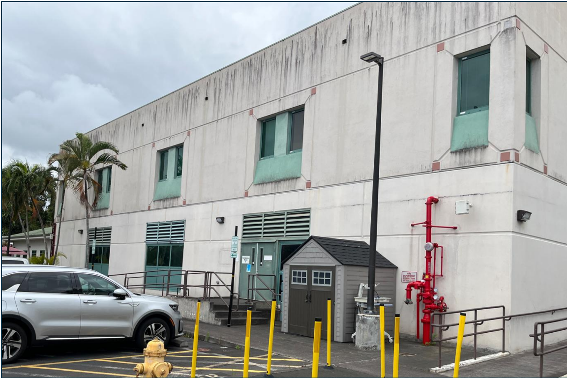
Photo 9 - Overview of Building 1 1998 addition typical exterior wall with EIFS cladding (West Elevation)
