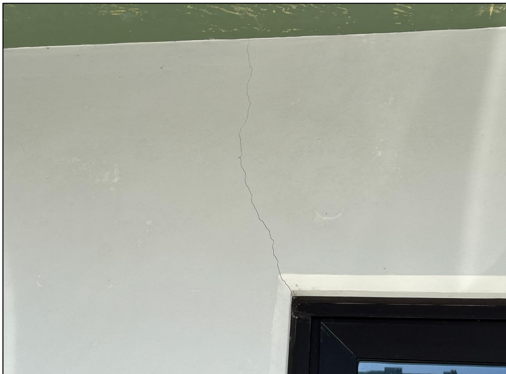
Photo 22 - Cracked concrete at window at east elevation of Building 2
