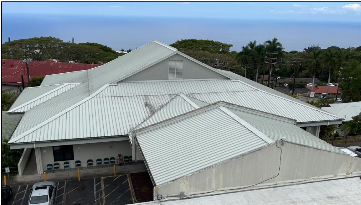
Photo 17 - Overview of standing seam metal roof at Building 2 and porte-cochere (view facing west)
