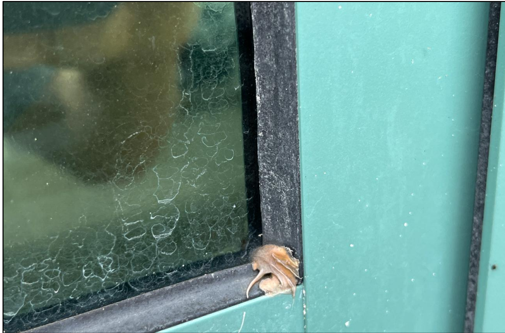
Photo 16 - Sealant repair at window glazing gasket noted at Building 1 1989 Addition West Elevation
