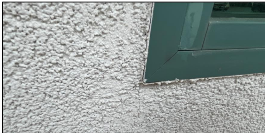
Photo 26 - Typical detailing at window and EIFS cladding. No sealant joint observed at window perimeters. Note touch up paint.
