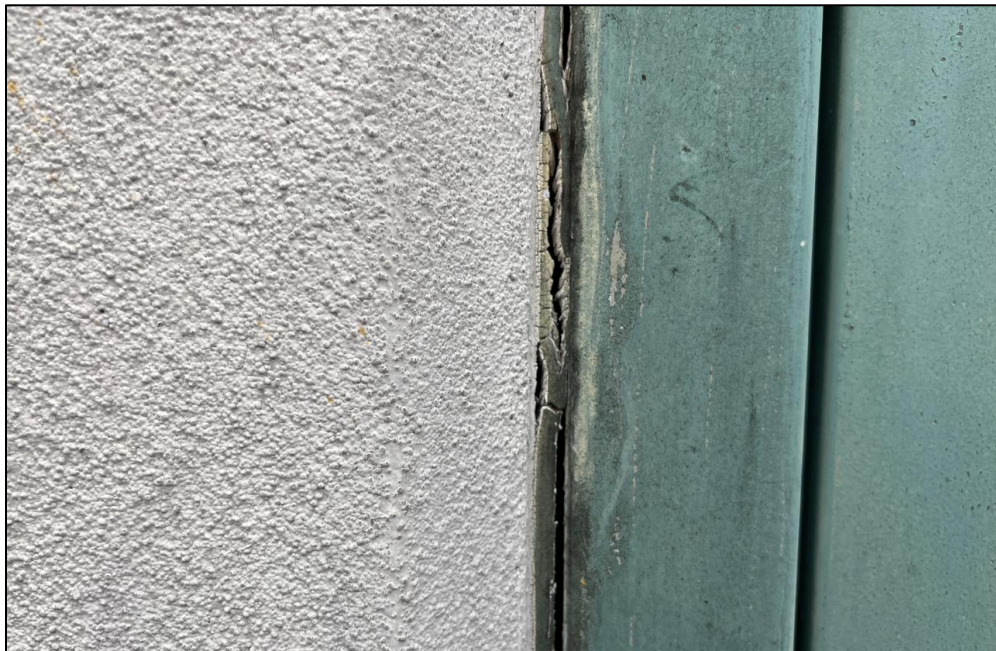
Photo 15 - Failing sealant joint between steel door frame and EIFS cladding at the West Elevation of Building 1 -1989 Addition
