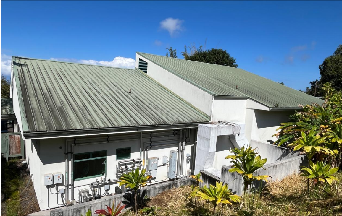
Photo 23 - Overview of Building 3 standing seam metal panel roof system viewed from east elevation
