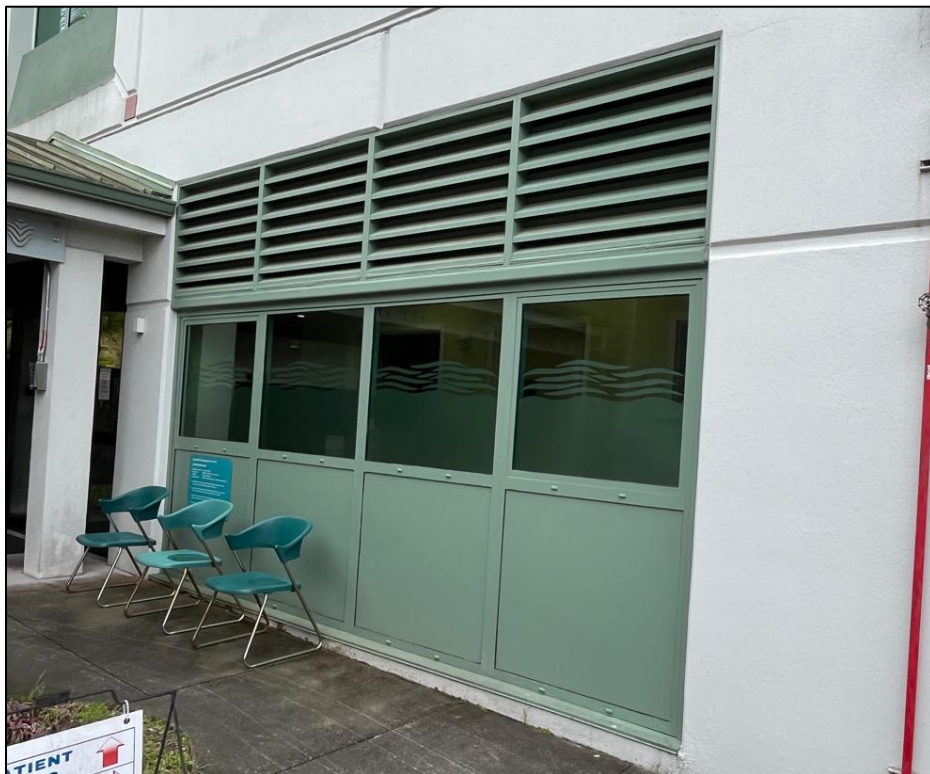
Photo 13 - Painted aluminum framed windows and painted steel louvers at Building 1 1989 Addition north elevation adjacent to Building 3.
