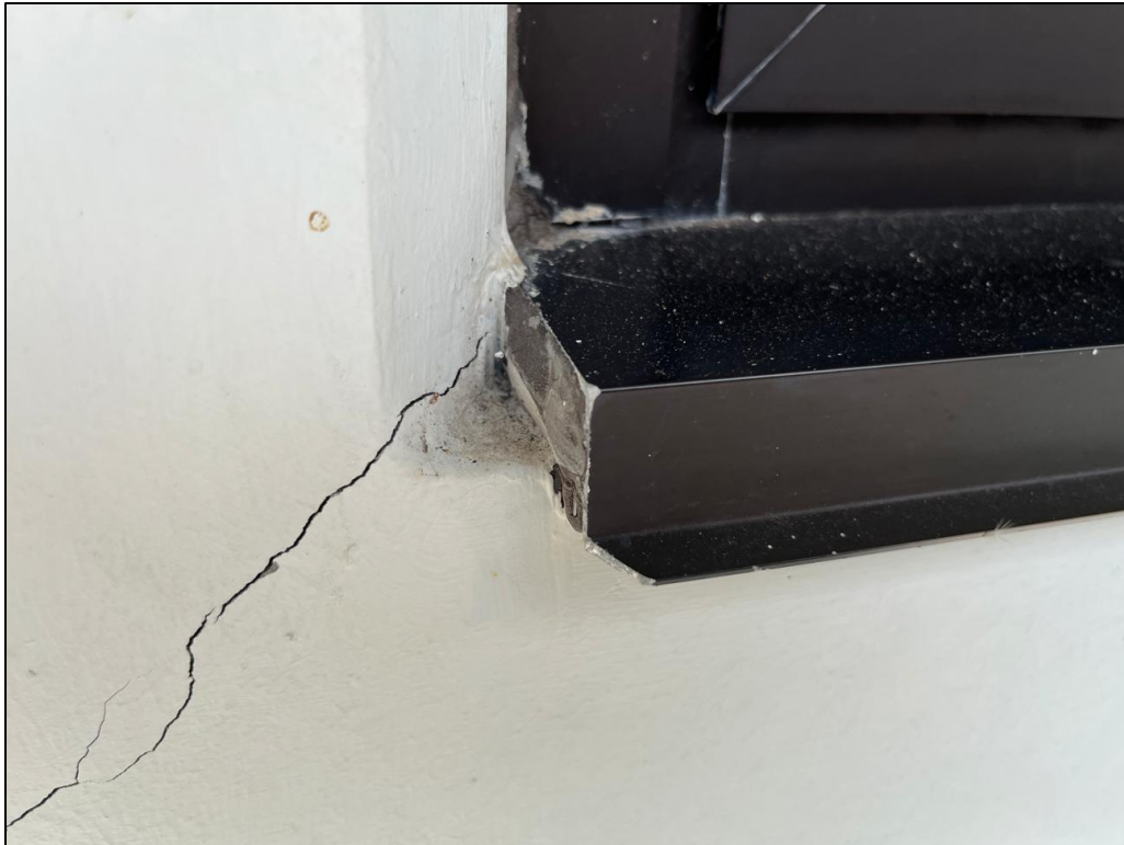
Photo 21 - Cracked concrete at window at east elevation of Building 2
