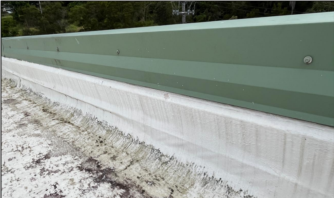
Photo 4 - Sheet metal coping over parapet wall and TPO membrane base flashing installed over counterflashing
