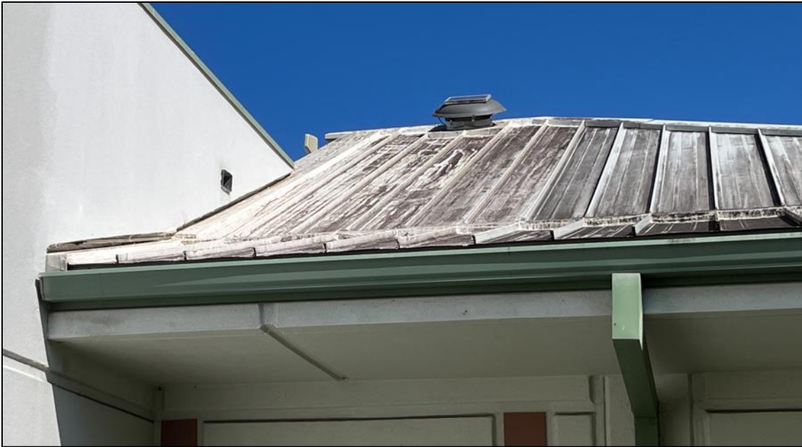
Photo 6 - Coating repairs at south elevation with improper detailing at roof sidewall flashing
