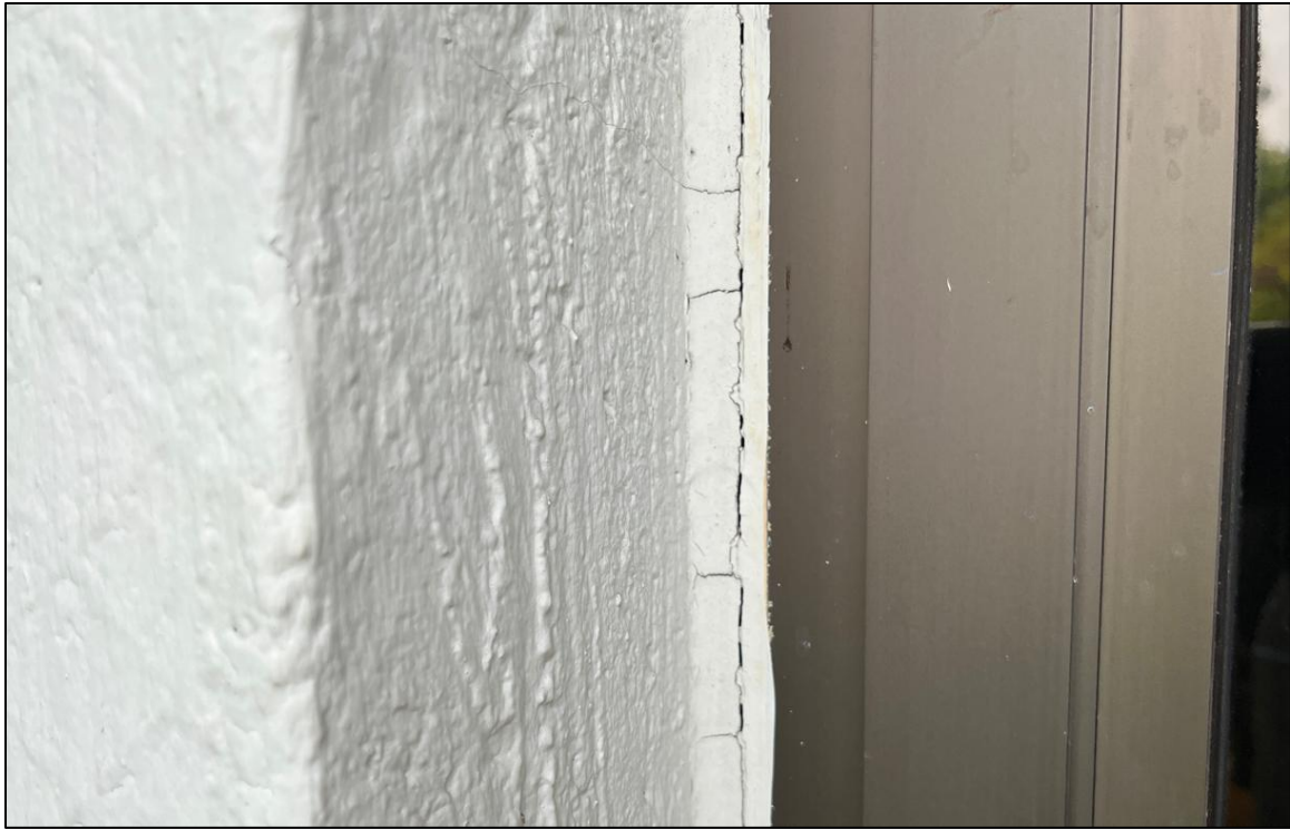
Photo 12 - Typical cracked paint finish applied over window perimeter joints
